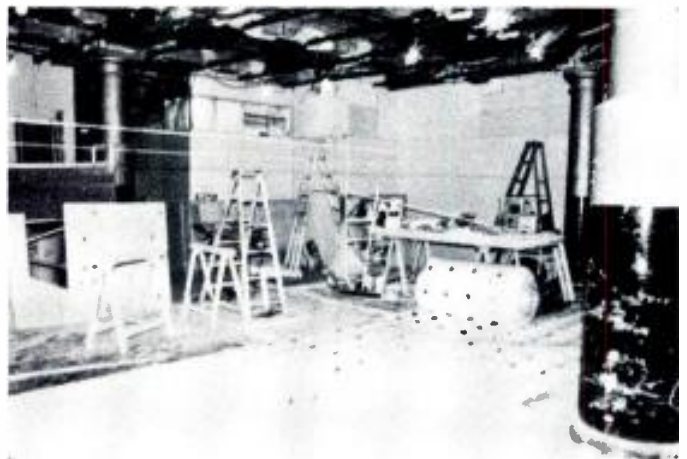
Flooring being laid—rubber isolators imbedded in fiberglass with a section of floor laid over it.
